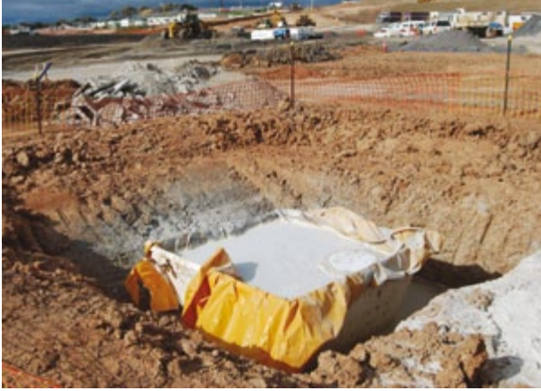
Excessive concrete pour recycling at Desal Plant
